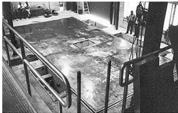
500,000 lb. Seismic Base under Construction. Base Size: 17 Ft X 25 Ft. X 8 Ft. thick.
